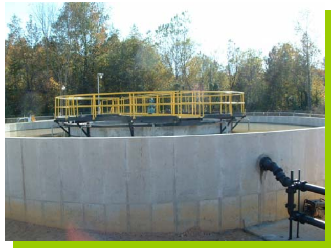
Typical Field-Erect Treatment System
